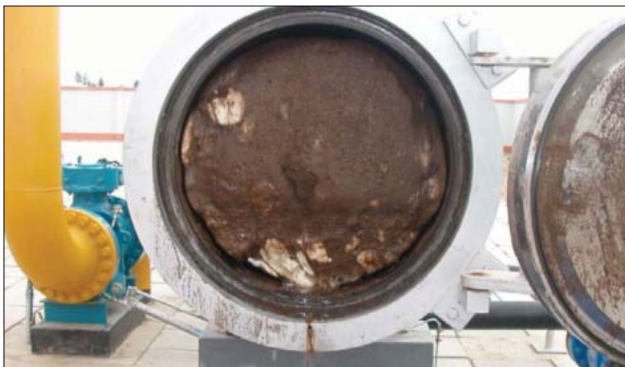
Operators of China's West-East Gas Pipeline found this ice-like object upon opening a pig receiver (Fig. 1).
